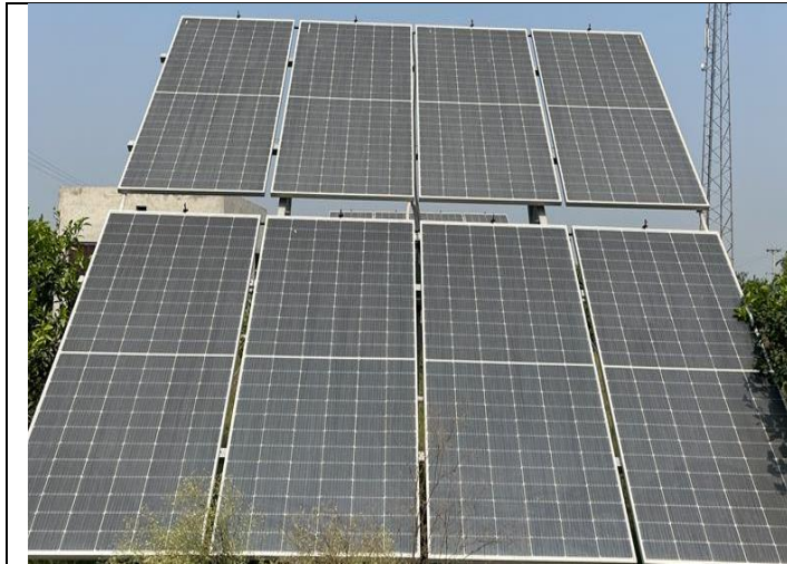
1-PV System for Irrigation
