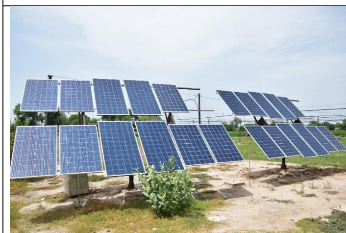
5-Solar System for irrigation (C-Block)
