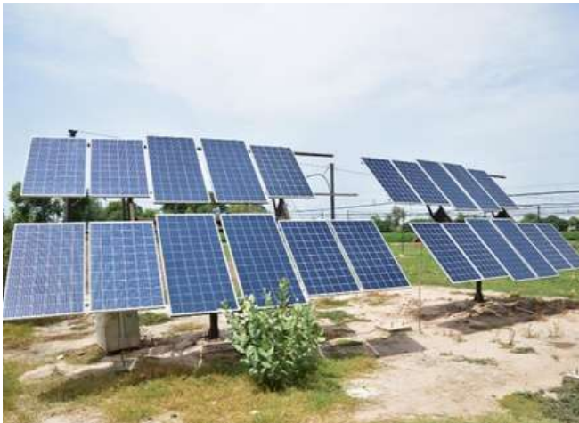
SOLAR SYSTEM FOR IRRIGATION IN C-BLOCK
