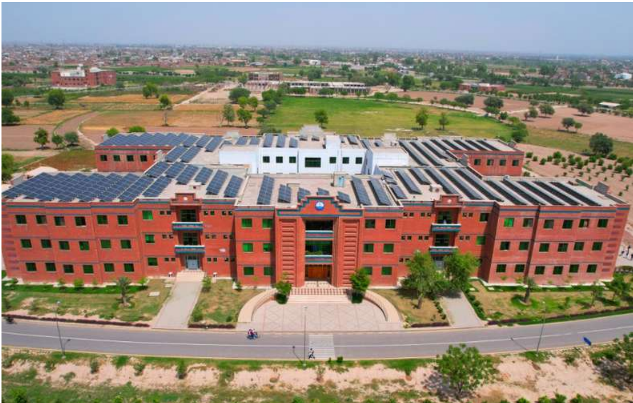
SOLAR POWER SYSTEM 500KW IN ACADEMIC BLOCK, MNSUAM
