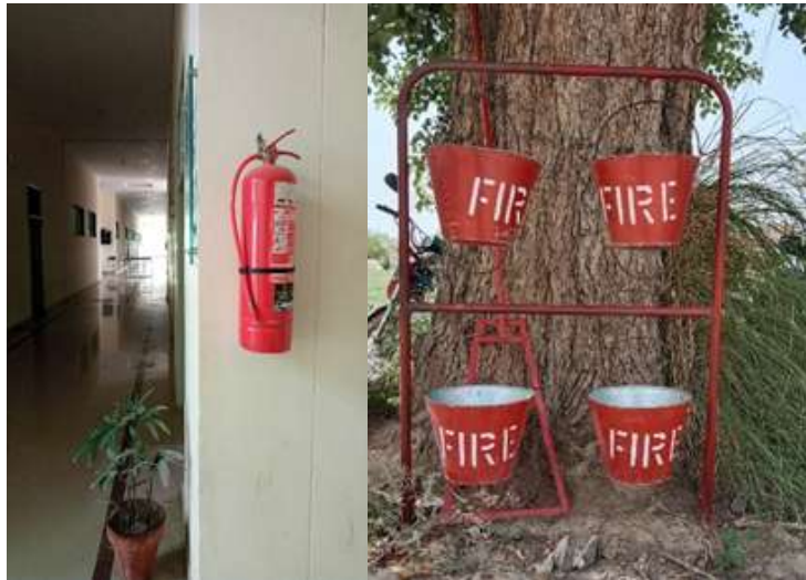
FIRE EXTINGUISHERS AND FIRE BUCKETS
